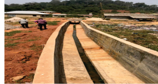
CONSTRUCTION OF 1.5M X 1.2M REINFORCED CONCRETE STORM WATER DRAIN (0.404KM) AND 0.6M U-DRAINS (0.35KM) AT SEFWI DWENASE MARKET
